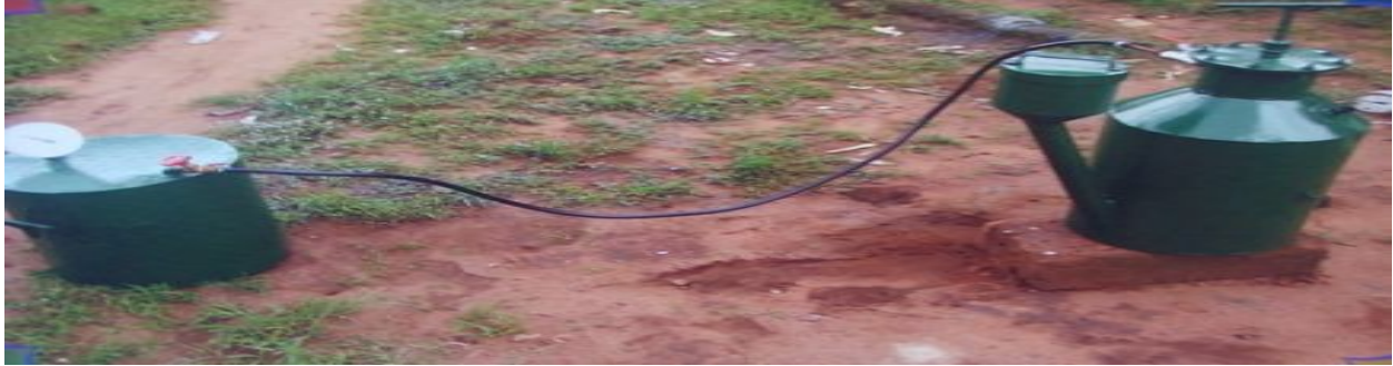
Plate 1: Simple Pilot Digester set up
